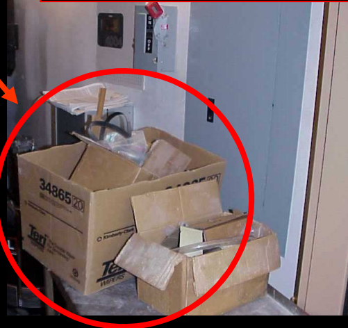
Improper Storage in front of Electrical Panel
